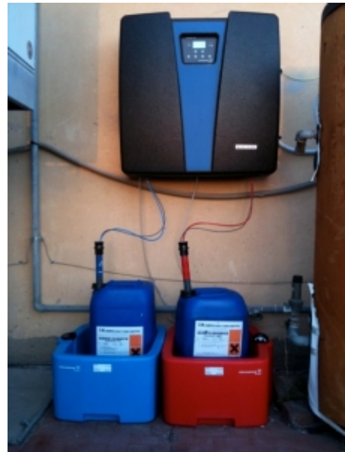
Oxiperm Pro system installed in hospital
